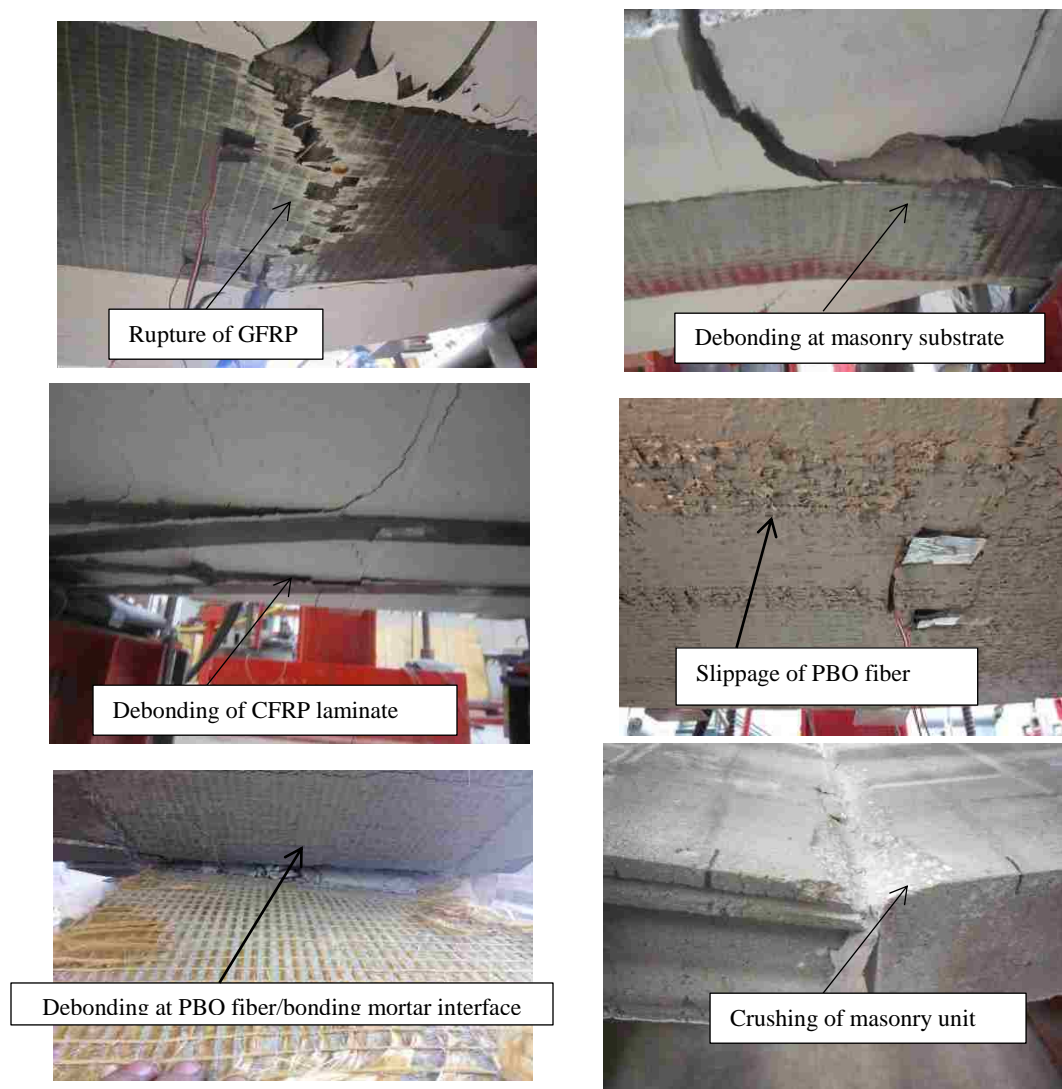
Figure 6. Typical mode of failures
