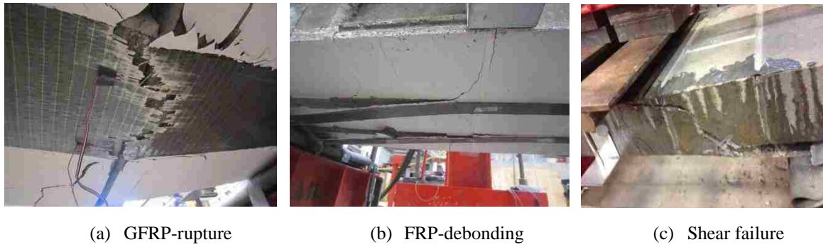
Figure 7. Observed modes of failure
