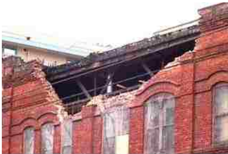
Figure 2.2. Failure of unreinforced wall due to out-of-plane seismic forces [Nisqually Earthquake, 28 February 2001].
